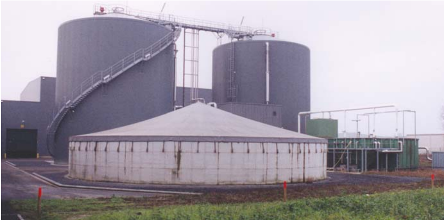
With its digesters and wastewater treatment system, the versatile renewable energy/composting facility in Belgium has capacity to process over 55,000 tons of MSW annually.
